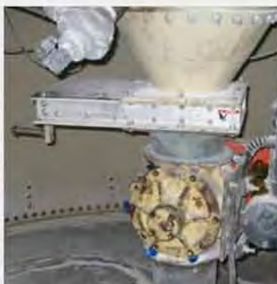
12" (305mm) Maintenance Gate above a rotary airlock handling soda ash
